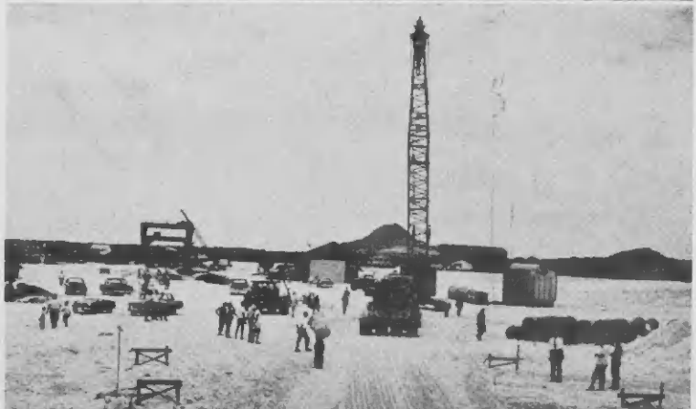
THE ENTIRE load is supported on forty-two wheels which keep the rig from sinking into the soft sand beach. Slowly, but surely, bottom photo, the rig moves toward the erection site. HENTER E carga ta wanta ariba cuarenta y dos wiel, cual ta tene e trailer pa e no staka den e santo moli di lama. Poco-poco e trailer ta bai na su lugar.
